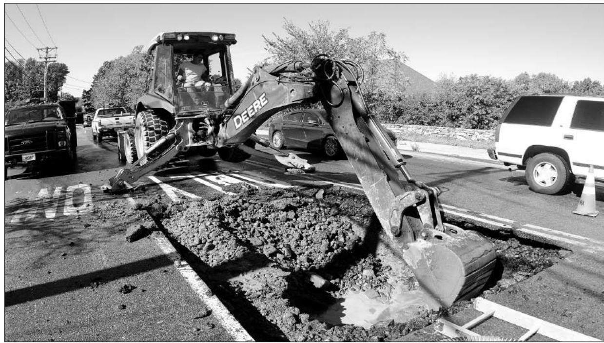
A worker digs on Chestnut Street near Metacom Avenue after a water main break Tuesday.
