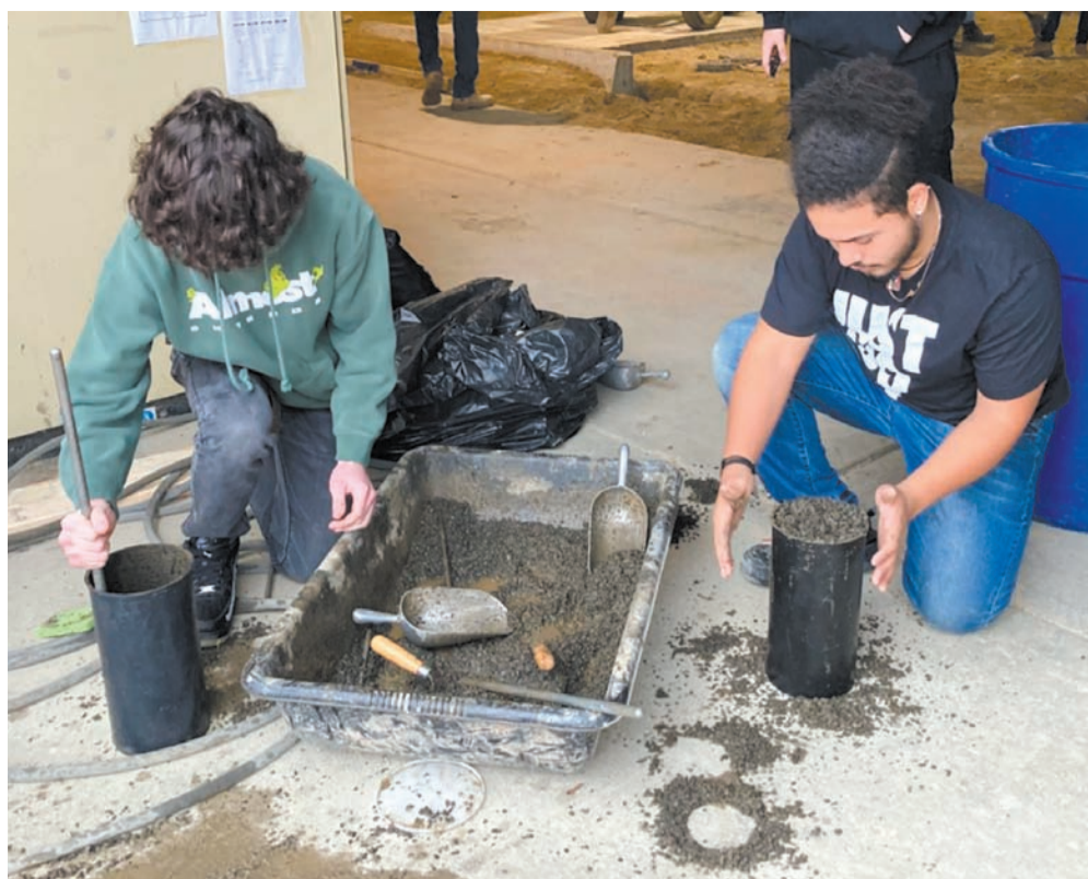
PRACTICE, PRACTICE, PRACTICE: After listening to Scott Zinke's instructions, Dylan Gibb & Ziaiah Dearce took turns packing concrete into cylindrical molds where they will later determine the strength of the concrete. (Herald photo)
